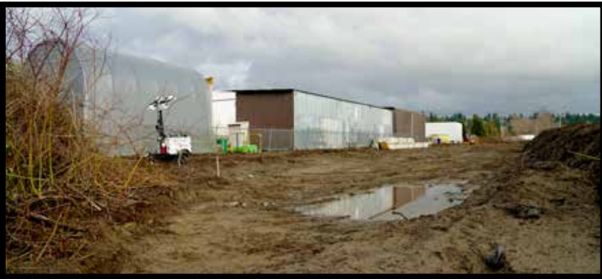
Below: The vegetation behind the Brenco property has been removed and will become a new roadway which is expected to open next year.
